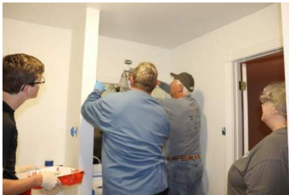
It took one to hold the light fixture while one painted the wall behind it.
