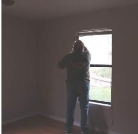
President Keith removed old blinds and readied window for the new ones.
